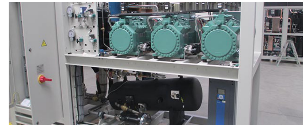
CO 2 - Cooled Units Used in Supermarkets
